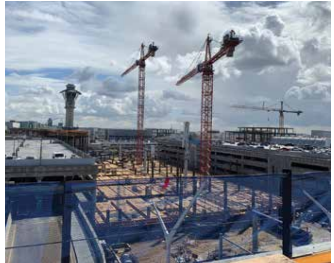
Los Angeles International Airport (LAX) – The $15 billion airport modernization program now underway at LAX is the largest public works program in the history of the City of Los Angeles. Photo by Wes Whittle.
